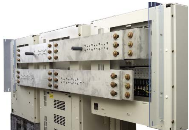
Copper Inter-bay Bus Bars (shown with cover removed for detail)
